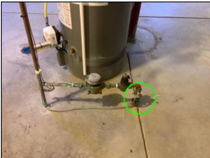
Comment: Water main shutoff
