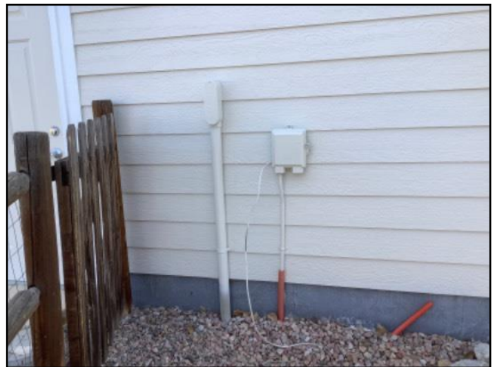
Comment: Service entrance to interior panel
