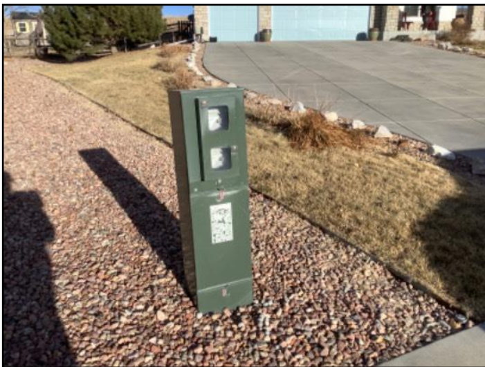
Comment: Service meter located near the end of the driveway
