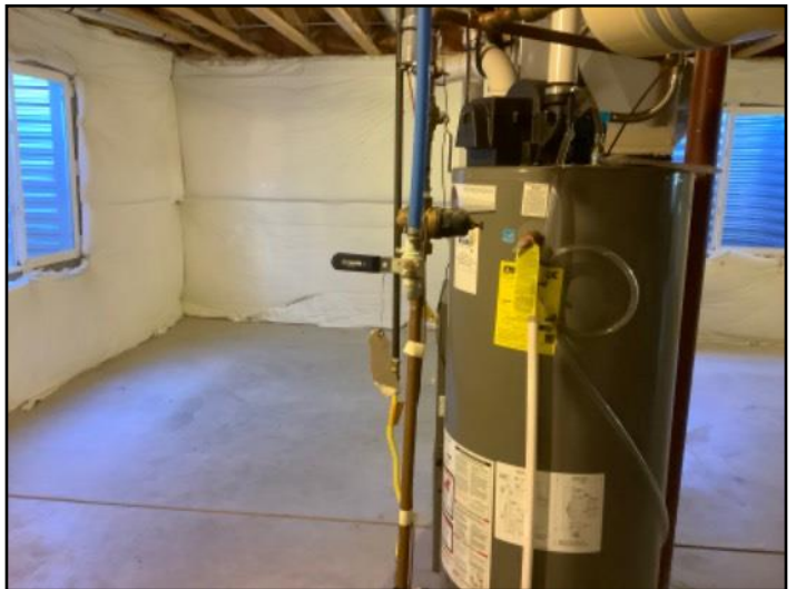
Comment: Sprinkler system shutoff valve
