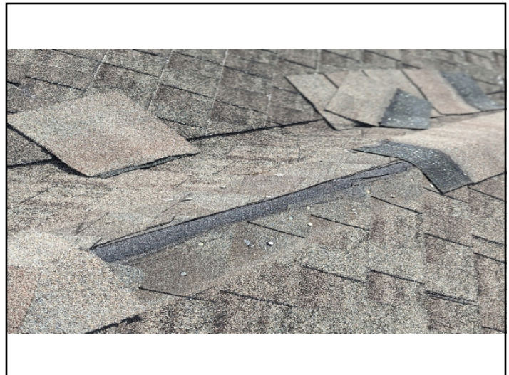
Comment: Damaged ridge cap
