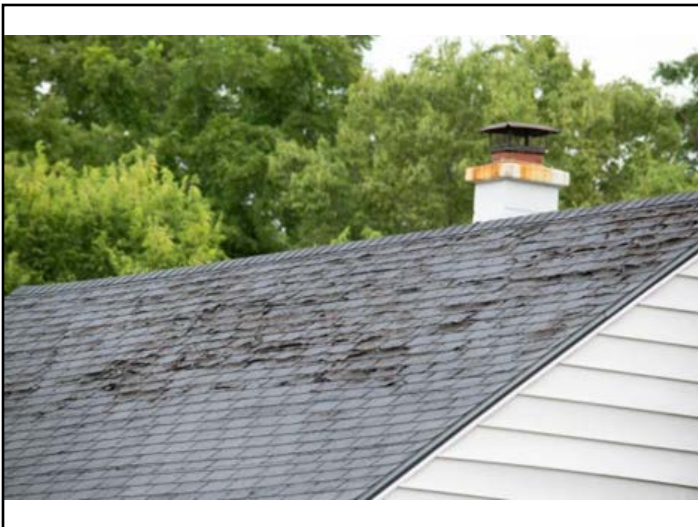
Comment: Heavily damaged section of roof
